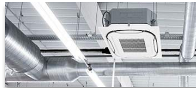
Hydraulic and pneumatic components (heating, ventilation, air conditioning, fire prevention/fighting, anti-pollution, etc.)
